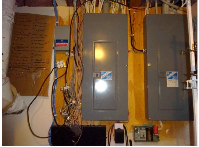
Electrical Service Entrance panel
