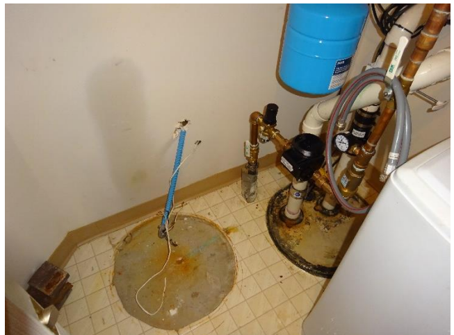
View of sumps in utility room
