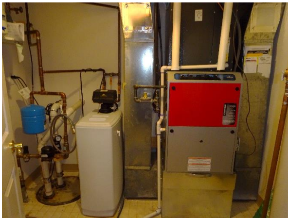
View of HVAC in utility room
