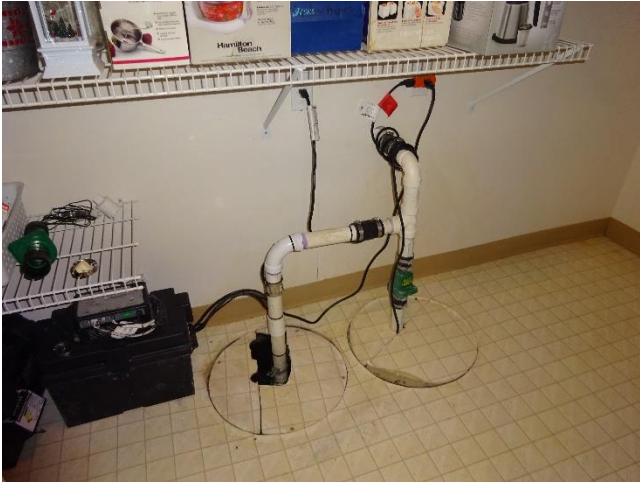
View of sump pumps in utility room
