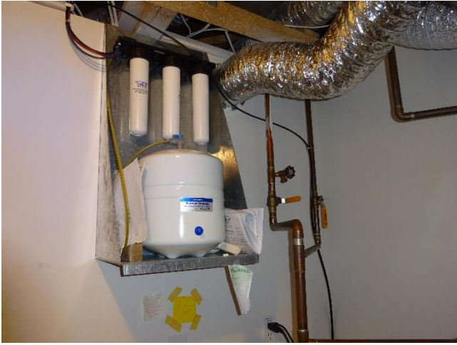
View of water treatment
